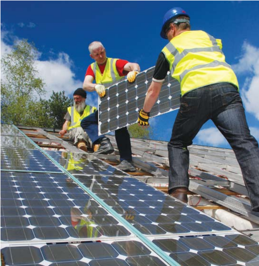
Photovoltaic roof – the Centre for Alternative Technology. Source: Centre for Alternative Technology.
